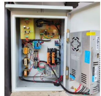
Fig. 8 Main Control Box
